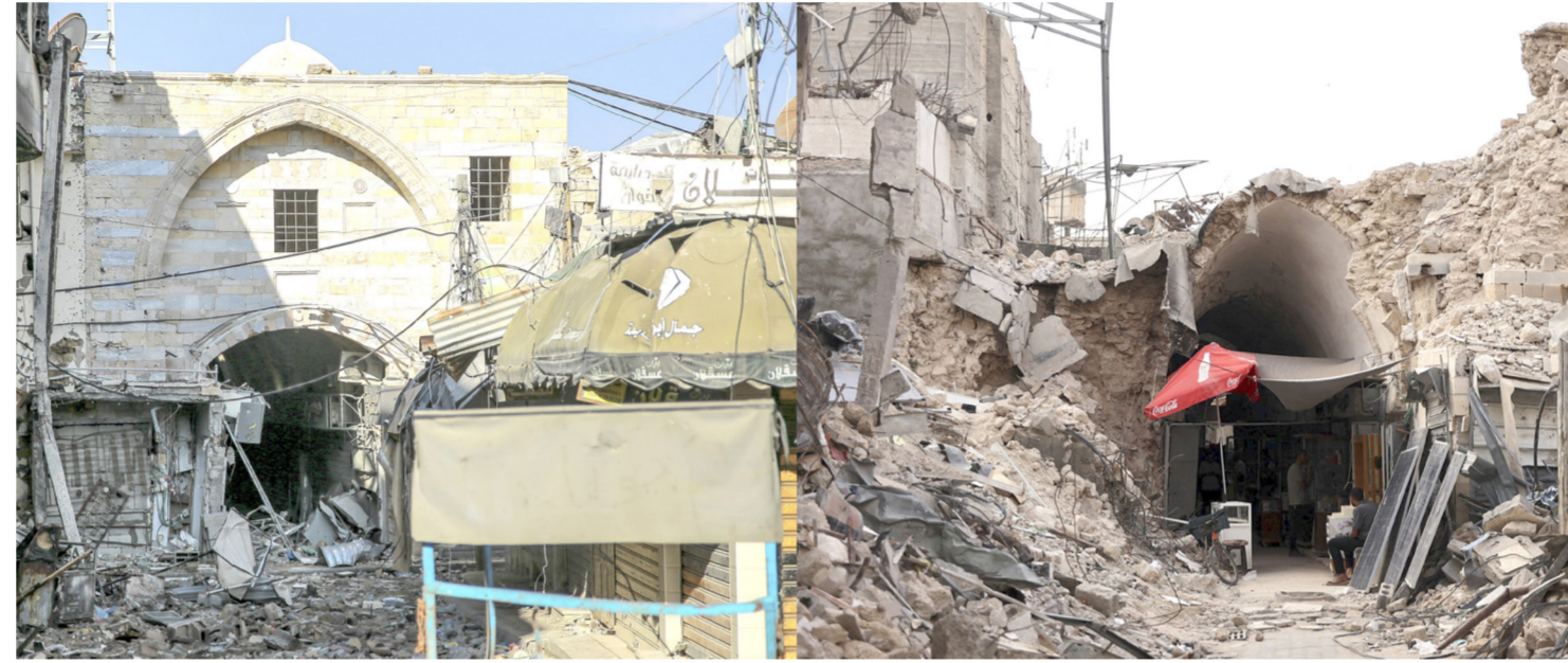
Gaza City's Qissariya Gold Market (Caesarea Market) after damage in Israeli bombardment on January 5, 2024; and (R) the same building after further damage on September 22; amid the ongoing war in the Palestinian territory between Israel and Hamas.
