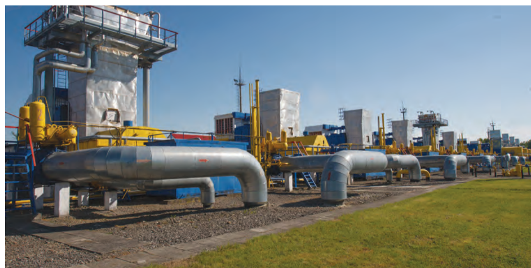
A view of pipelines at the Bilche-Volytsko-Uherske underground gas storage facility, the largest in Europe, not far from the village of Bilche village, in the Lviv region of western Ukraine
