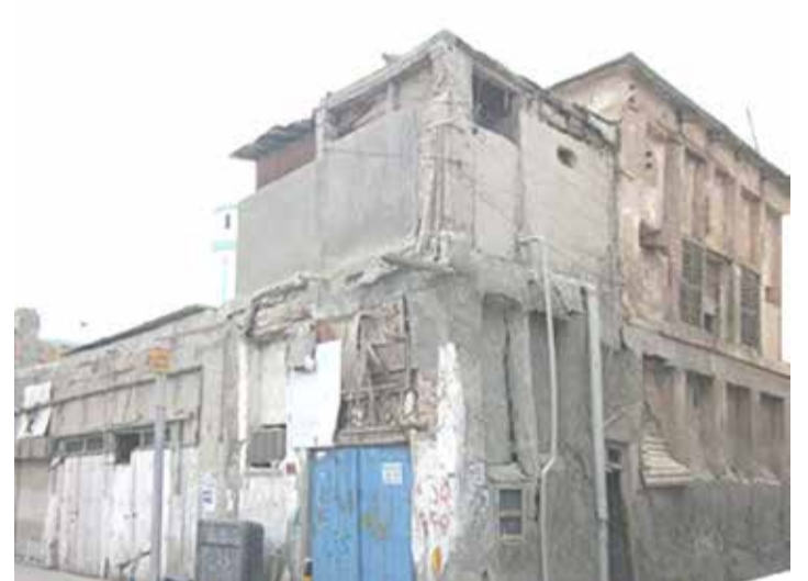
Dilapidated house in Muharraq
