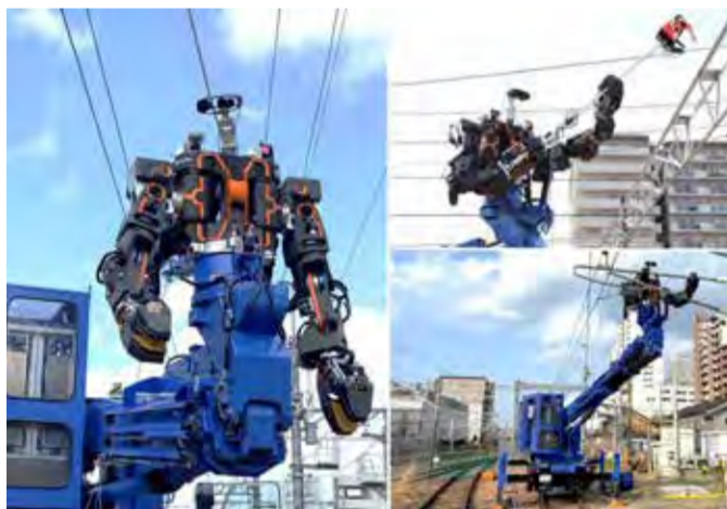
For now, the robot's primary task will focus on trimming tree branches along rails and painting metal frames that hold cables above trains
