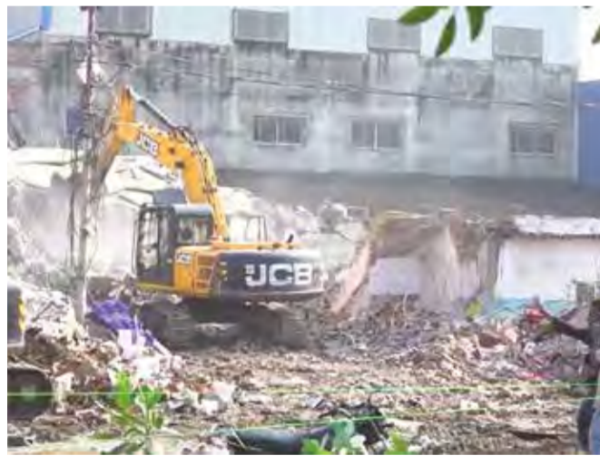
The commercial building, which had been used by multiple small companies -- including as a warehouse and as a vehicle workshop -- collapsed on Saturday afternoon.
