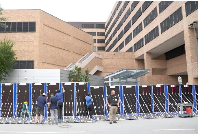
An AquaFence flood wall is put into place around Tampa General Hospital ahead of Hurricane Milton's expected landfall
