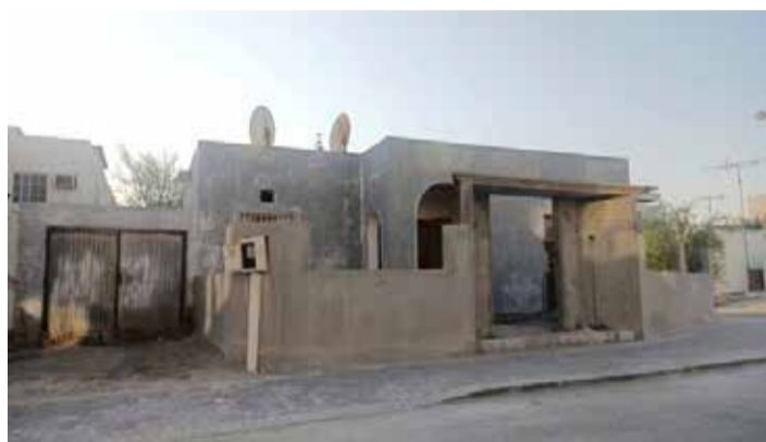
Abandoned buildings left in a state of disrepair
