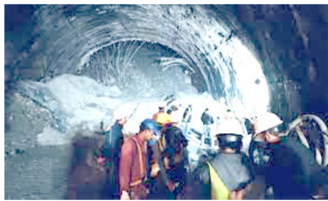
Rescue teams working to remove huge piles of concrete blocking the tunnel
