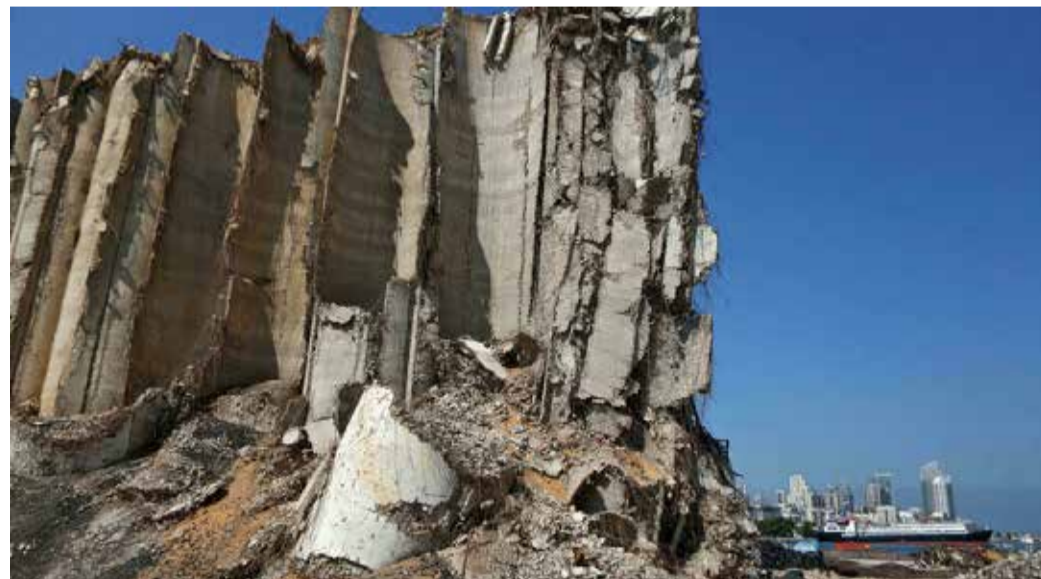
Damaged grain silos at the port of the Lebanese capital Beirut, almost a year after the August 4 massive explosion that killed more than 200 people
