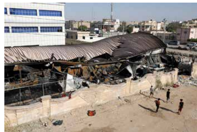
People walk past the damaged al-Hussain coronavirus hospital
