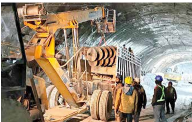
Rescue workers at the site after a tunnel collapsed in the Uttarkashi district of India's Uttarakhand state
