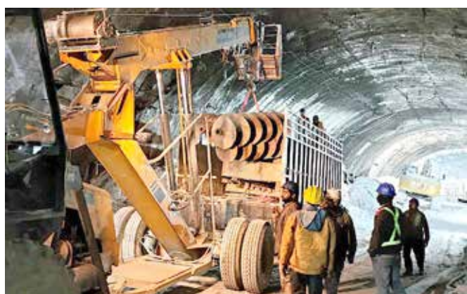
Rescue workers at the site after a tunnel collapsed in the Uttarkashi district of India's Uttarakhand state
