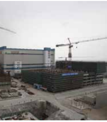
part of the Taishan Nuclear Power Plant, or Power (CGN), is seen under construction 7, 2013.
