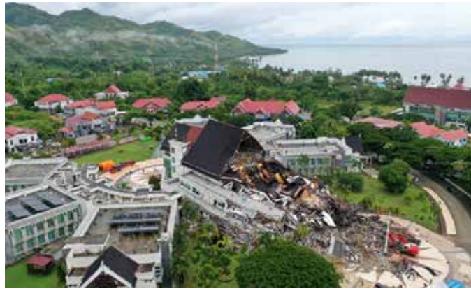
An aerial picture shows damaged office of the governor of West Sulawesi province following the earthquake AFP | Jakarta
