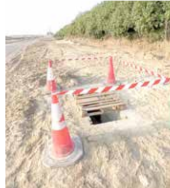
An open manhole in the Northern Governorate
