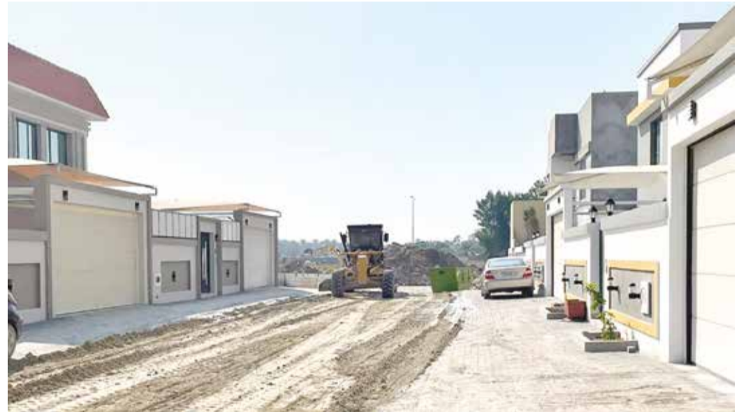
The Ministry of Works yesterday announced that it is currently carrying out levelling works of roads in Block 1038 in the Sadad area. The road, ministry said, will be paved with asphalt after the construction of the sewage network, which is in the final design stage. Implementation is approved according to the priority determined by the project's technical readiness, the region's rate of reconstruction, and the availability of financial funds.
