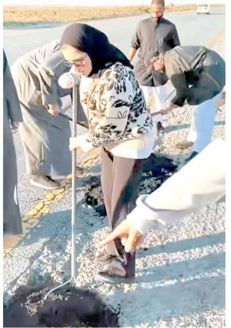
Kuwaiti citizens patch up the potholes to avoid another accident
