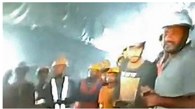
A group of workers trapped inside the under-construction tunnel, days after it collapsed in the Uttarakashi district of India's Uttarakhand state
