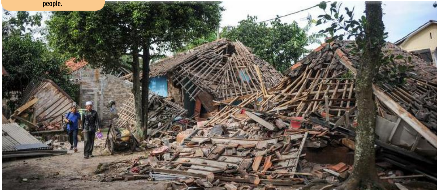
Locals walk past collapsed houses after an earthquake in Cianjur, West Java province, Indonesia
