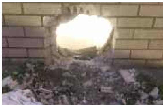
They used makeshift tools to take advantage of a construction flaw
