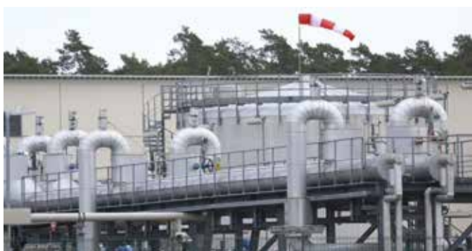
A wind gauge flutters over the landfall facility of the Baltic Sea gas pipeline Nord Stream 1 in Lubmin, Germany
