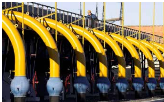
A worker checks pipes at a gas compressor station on the Yamal-Europe pipeline near Nesvizh, some 130 km (81 miles) southwest of Minsk
