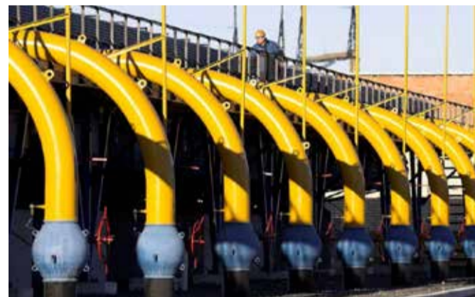
A worker checks pipes at a gas compressor station on the Yamal-Europe pipeline near Nesvizh, some 130 km (81 miles) southwest of Minsk
