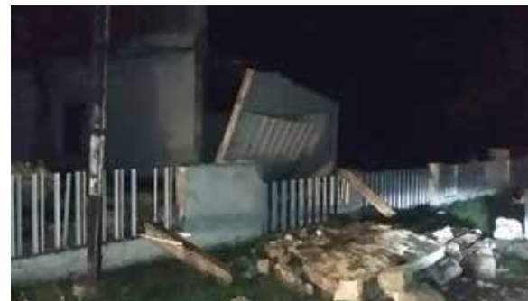
The collapsed wall of a building after the earthquake
