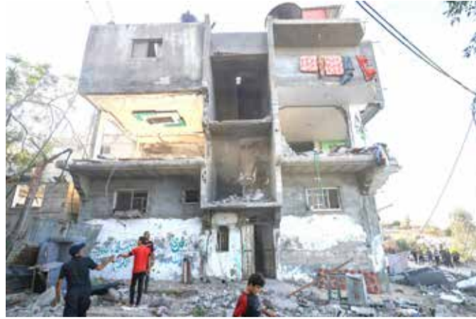
Palestinians search a damaged building following Israeli strikes in Khan Yunis in the southern Gaza Strip
